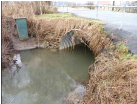
(a) Upstream end of newly replaced culvert on Stoney Creek at Bateman Road
