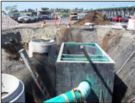
Oil Grit Separator
