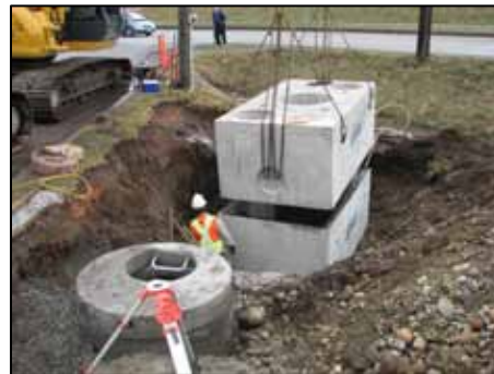
Oil Grit Separator
