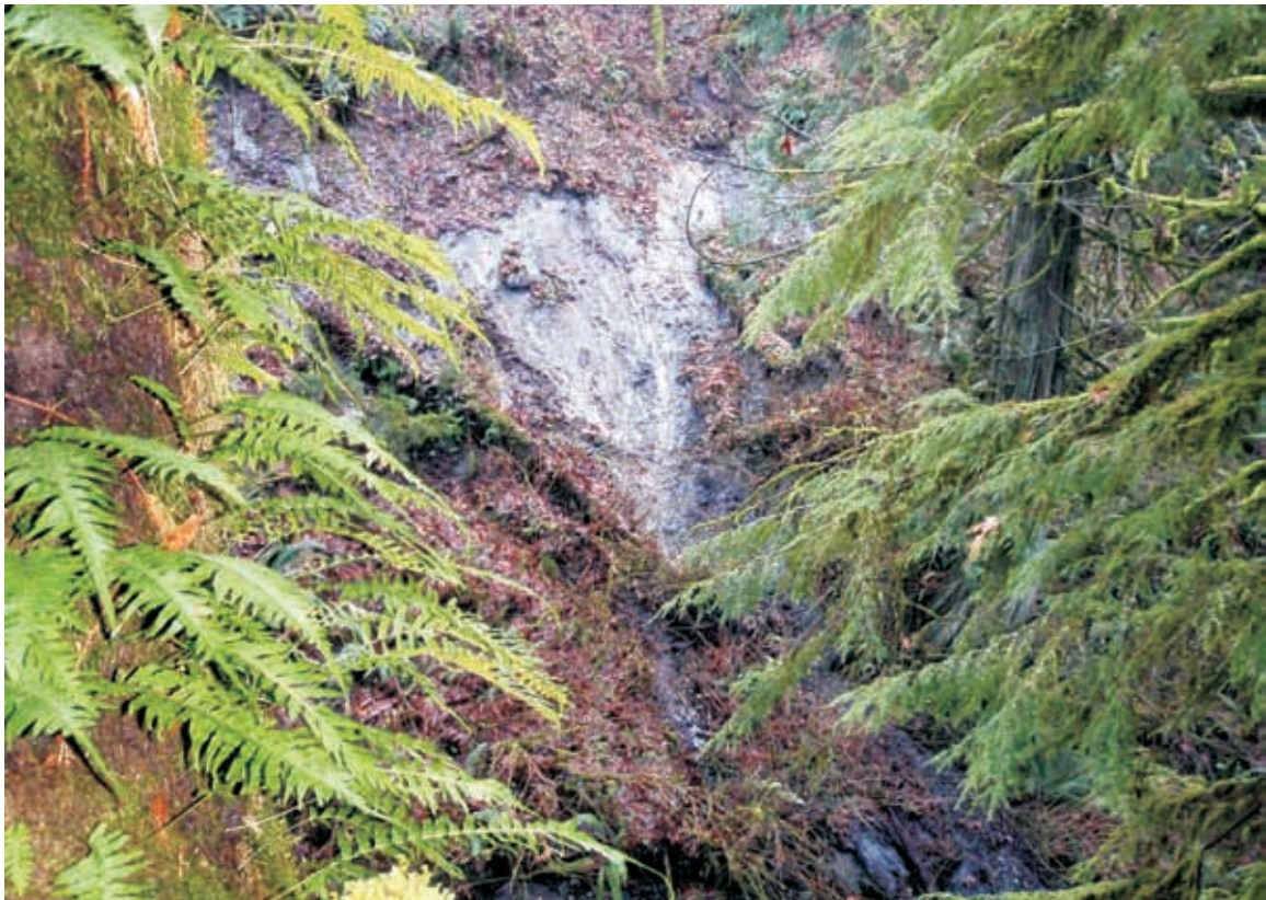
Photo 12. View of recent debris slide on lower ravine slope immediately above Clayburn Creek.
