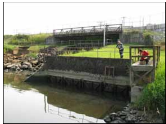
(b) Dyke floodboxes and flapgates (downstream side)
