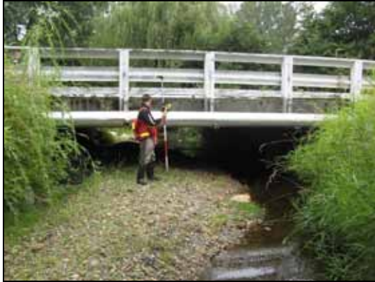
Photo 1-11: Sedimentation under Wright Street Bridge
