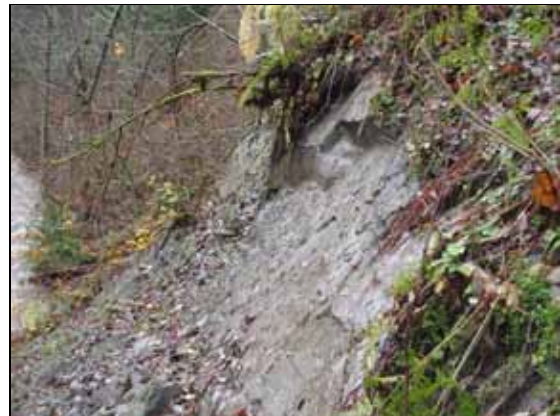
Photo 5-2: Debris Slide on Lower Ravine Slope
