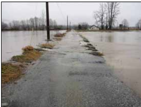
Photo 1-5: Overtopping and Erosion of Driveway 34416 Clayburn Road Dec. 2010
