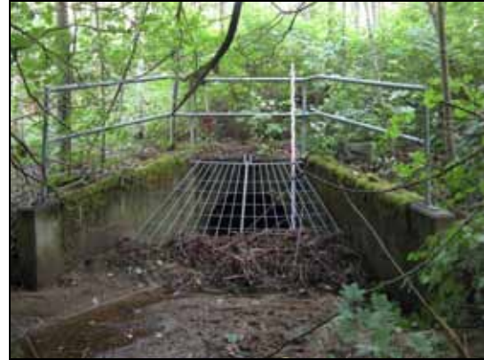
Photo 1-12: Debris on Trash Rack
