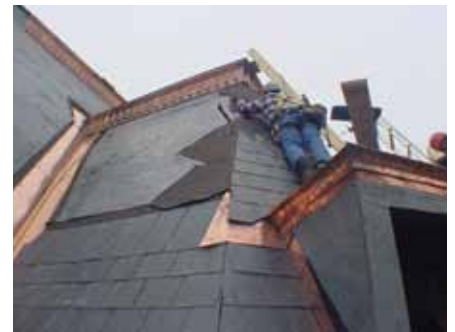
The Rehabilitation of the Truro Post Office, in Truro, NS included restoring its distinctive slate roof. In Rehabilitation, the replacement of missing historic features with a replica based on physical and documentary evidence, as in this project, is acceptable, as is a new design that is compatible with the heritage value of the historic place.
