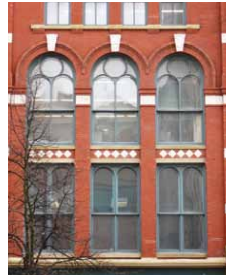
These large windows on King Street in St. John were originally slated for removal and replacement as part of the CentreBeam Place rehabilitation project. Instead, a condition revealed that the original windows could be retained and repaired, with the addition of interior storm to meet energy efficiency requirements.
