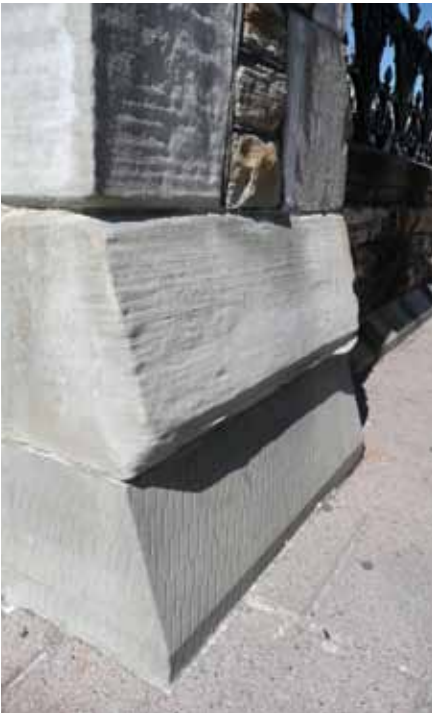
The new pieces of stone on the Wellington Wall at the Parliament Grounds in Ottawa are clearly visible on close inspection due to a different tooling technique.
