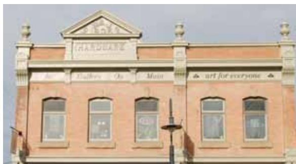
The two remaining decorative sheet metal urns at the top of the façade of the M & J Hardware Building in Lacombe, AB were determined to be beyond repair due to weathering over time. A third sheet metal urn (centre) was missing. The existing deteriorated elements and photographic documentation were used to replicate these elements. The M & J Hardware Building is an example where missing features from the restoration period have been re-instated based on physical and documentary evidence.
