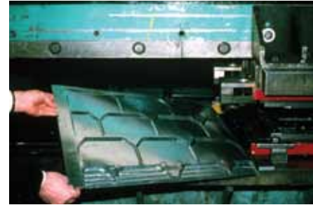
A surviving pressed metal shingle was used as a prototype for manufacturing replacement shingles when restoring the main house at the Motherwell Homestead near Abernathy, SK. In Restoration, repairs or replacements of extensively deteriorated or missing parts of features are done in kind, and are based on physical, documentary and oral evidence.
