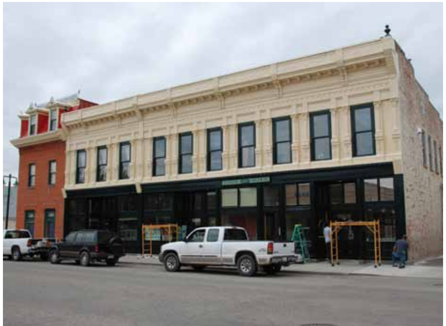
East façade after restoration of storefronts and preservation of pressed metal façade. Maintenance (repainting) in progress.
