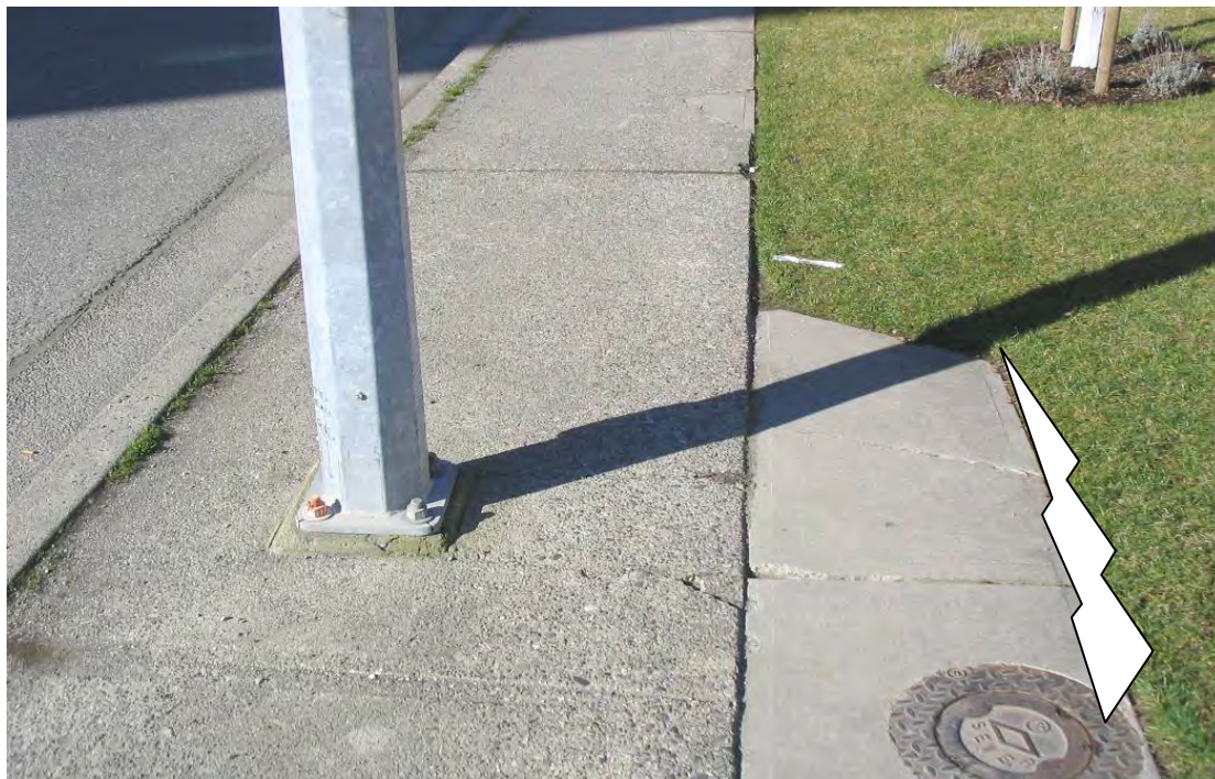
Figure 64: Pole in sidewalk, sidewalk widens, uneven surfaces..
