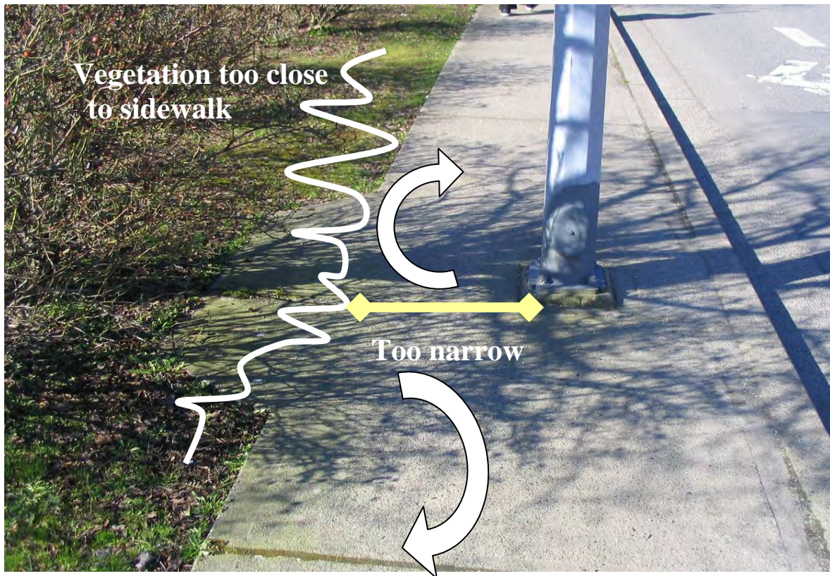
Figure 67: Widen sidewalk around pole. Vegetation causes an obstruction.
