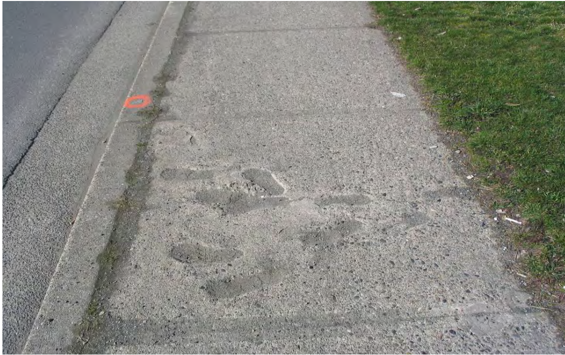
Figure 70: Rough sidewalk surface.
