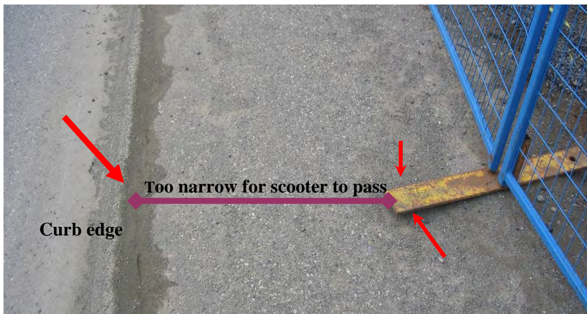
Figure 55: Obstruction on sidewalk. Potential to damage scooter wheels. Not enough room to pass. Passing obstacle would be too close to curb edge.
