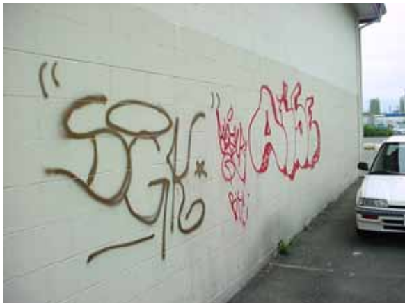
Figure 6. Large, blank walls attract graffiti.
