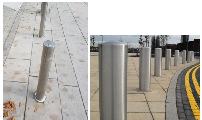
Example of Stainless Steel Bollards
