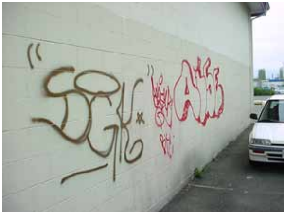
Figure 6. Large, blank walls attract graffiti.
